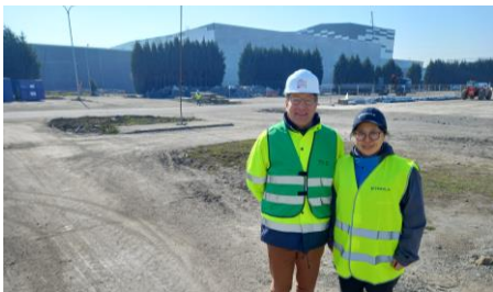
Standing in the foreground of the Billy-Berclau gigafactory: Pierre-Alain Dufour, ACC Launch Team Manager of the plant and Ma Jing, SEGULA Technologies Cell Assembly referent interpreter. (©SEGULA Technologies)
